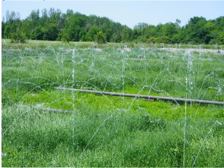
Treated waste water being applied to the intermittent sand filters.
