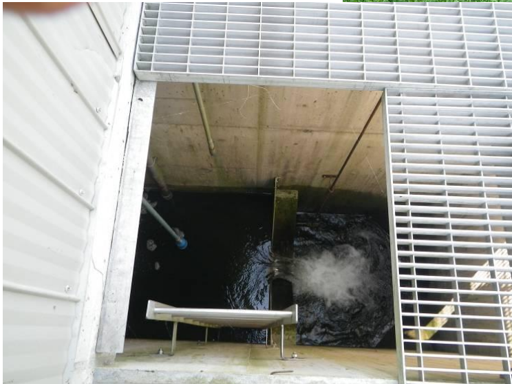
Under drainage from sand filters passing through V-notch weir.
