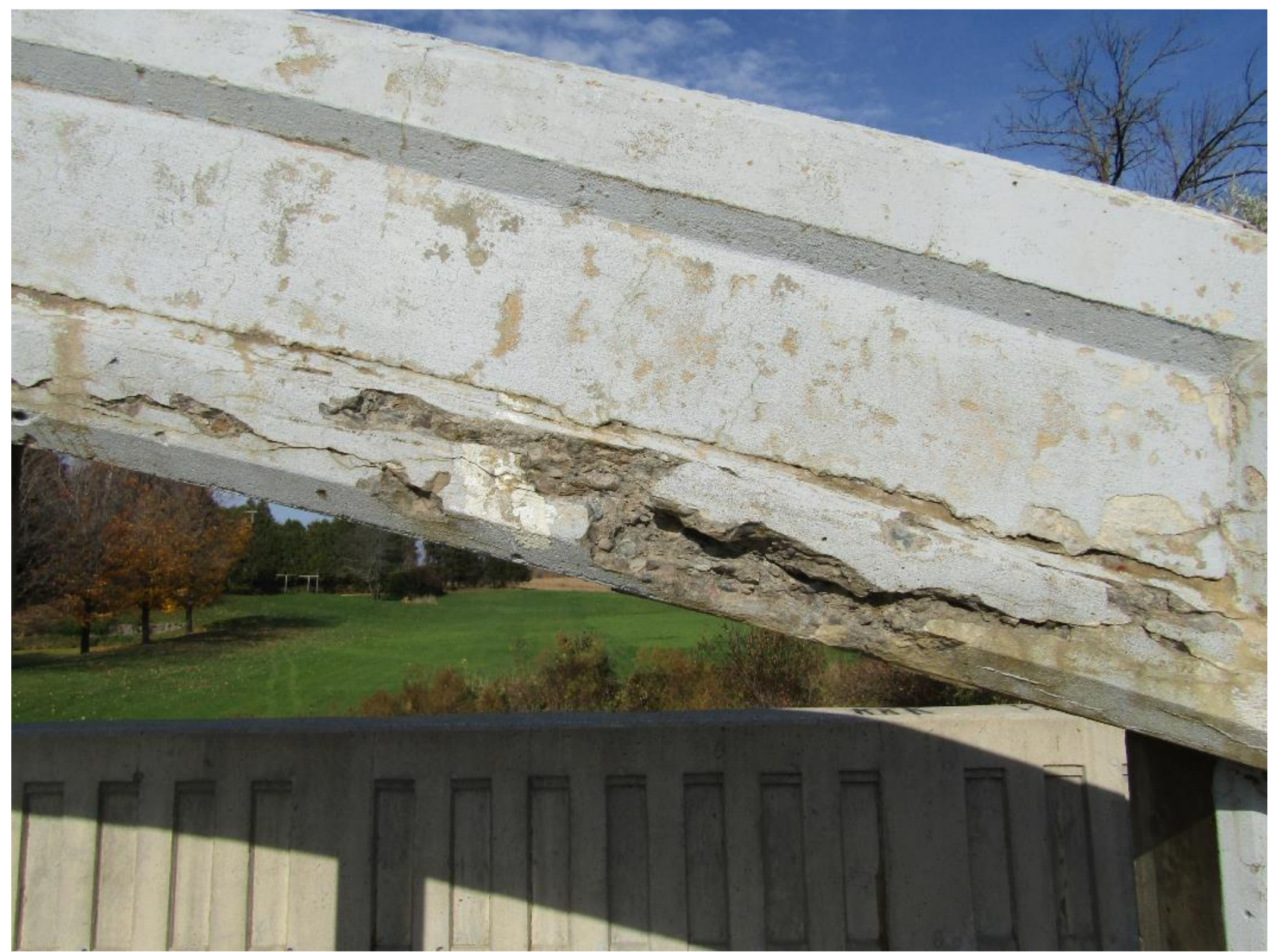
SPALLING ON NORTH ARCH
