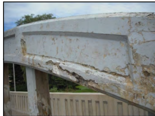
SPALL ON NORTH ARCH
