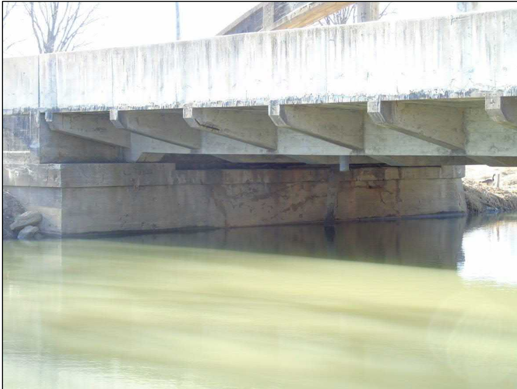
Image 26: Detail showing concrete abutments and cantilevered sidewalk on north side of the bridge
