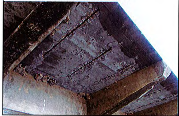
SPALL WITH EXPOSED REBAR CLIFF SWALLOW NESTS
