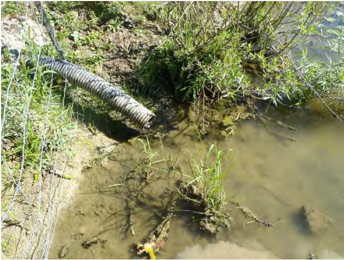
Photo 9: Overflow pipe from the Pond
