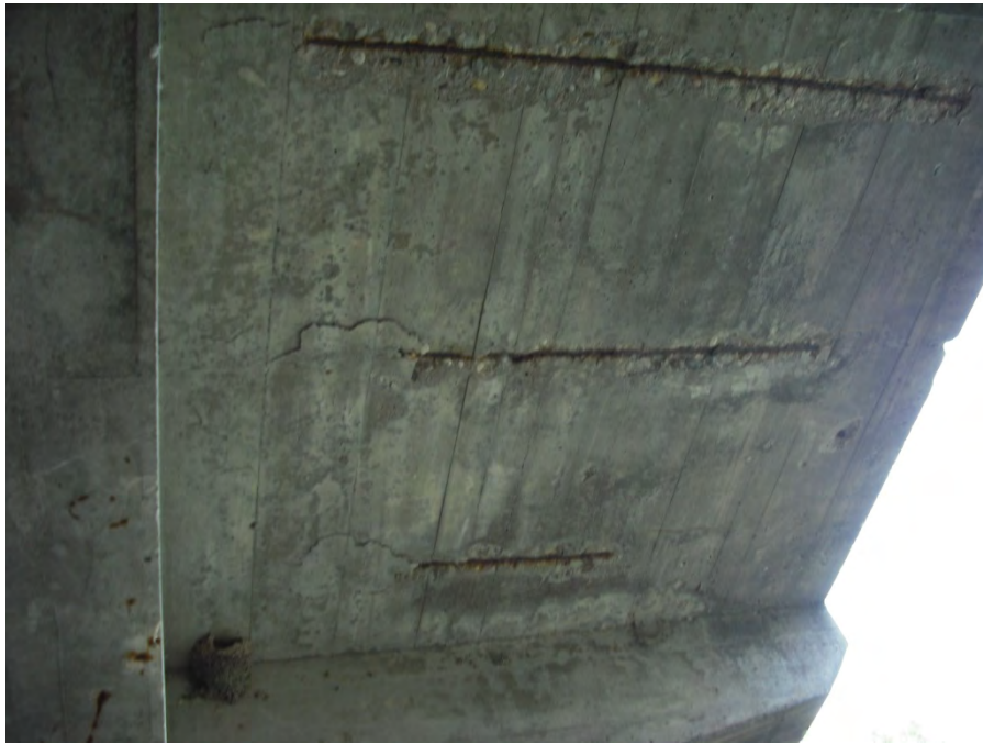
Spall with exposed rebar
