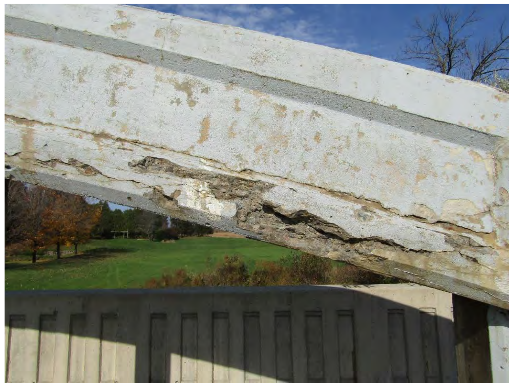
SPALLING ON NORTH ARCH
