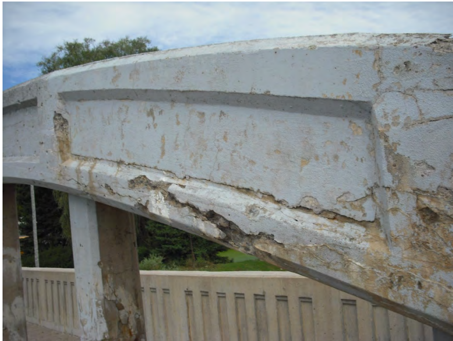
Spall on north arch
