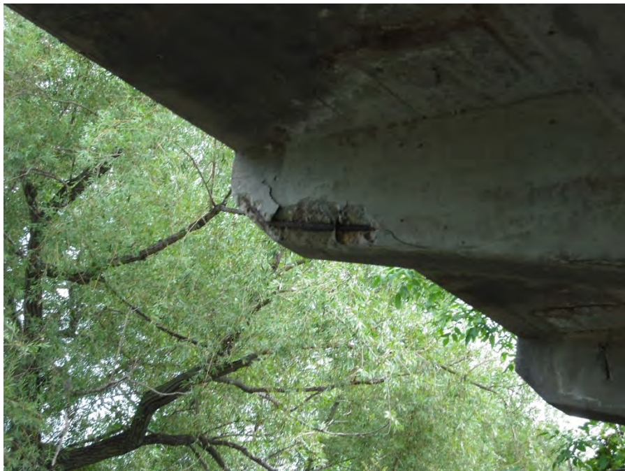
Spall with exposed rebar
