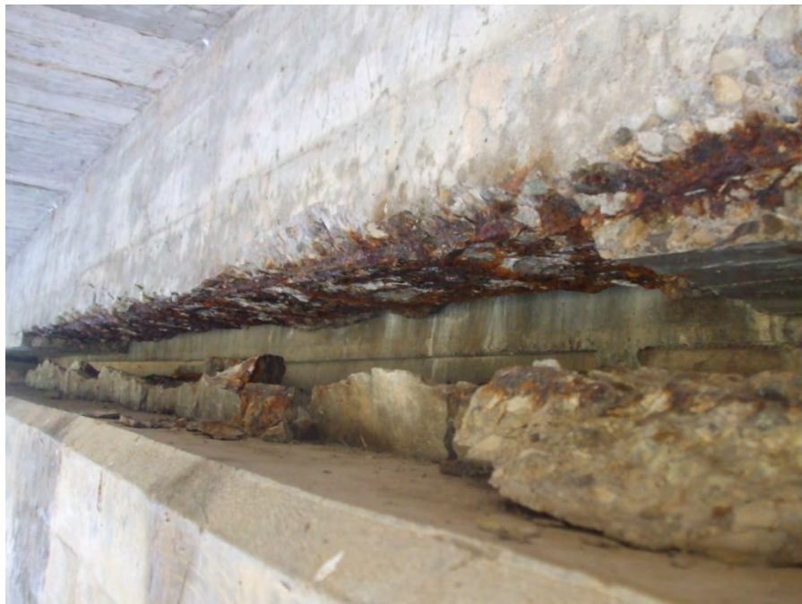
Severe spall with exposed rebar - east floor beam
