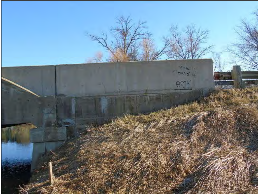
Image 16: View showing concrete abutment, guardrail and earthworks on the east side of the bridge
