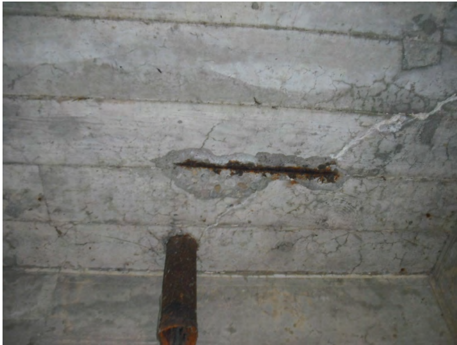
Spall with exposed rebar
