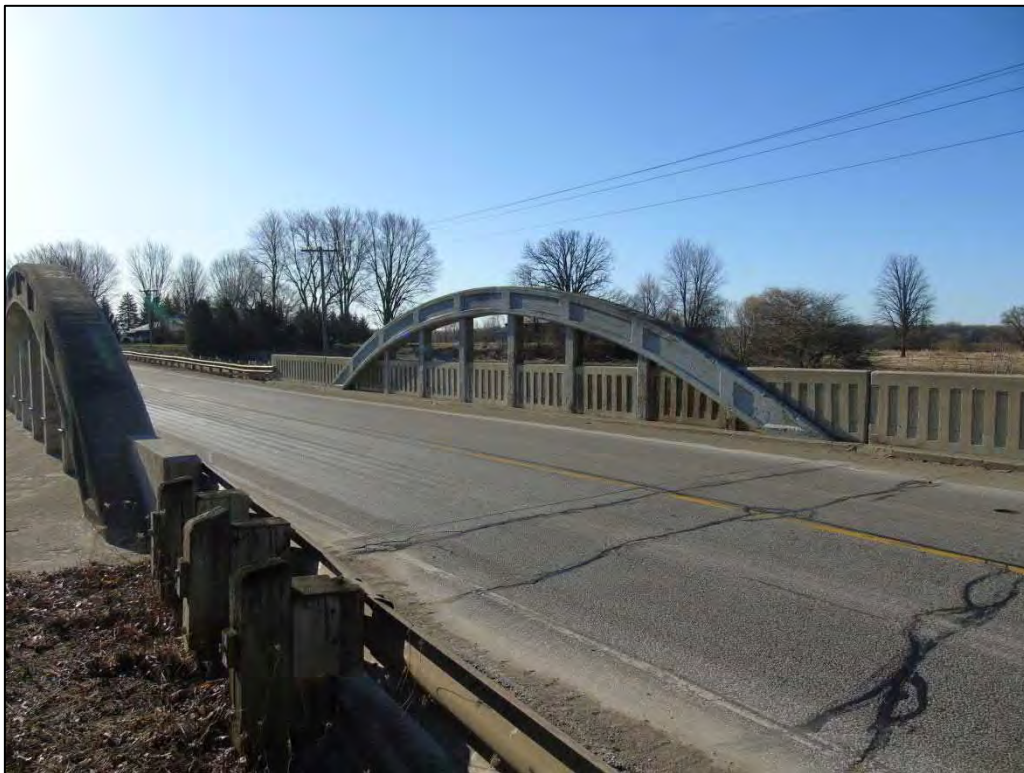
Image 17: View looking across County Road 22/Egremont Road showing bowstring arch and concrete guardrail
