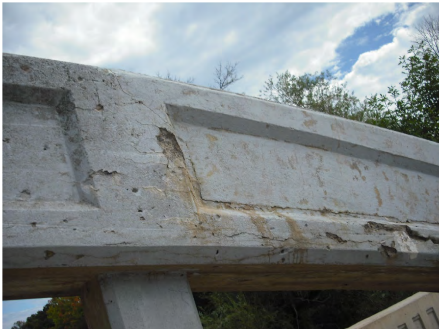
Spall on north arch
