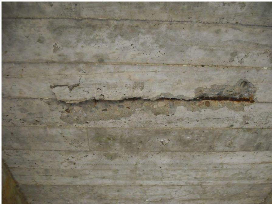
Spall with exposed rebar
