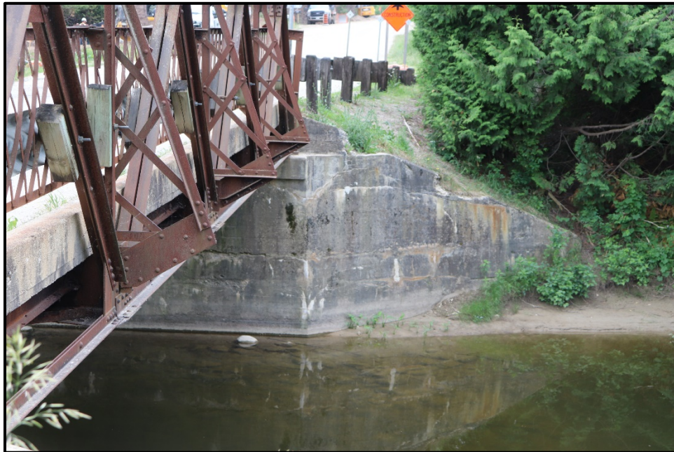
Image 7: Detail of south abutment and wingwall showing deteriorated concrete (TMHC 2020)
