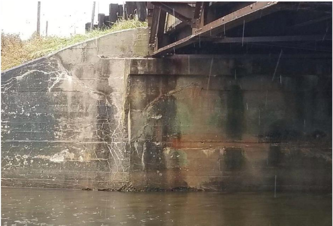
Figure 2.7 Cracked Ballast Wall and Abutment
