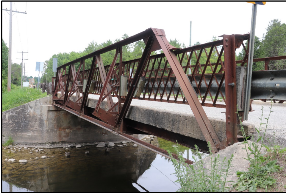
Image 4: Truss and railing on east side of structure and south abutment (TMHC 2020)
