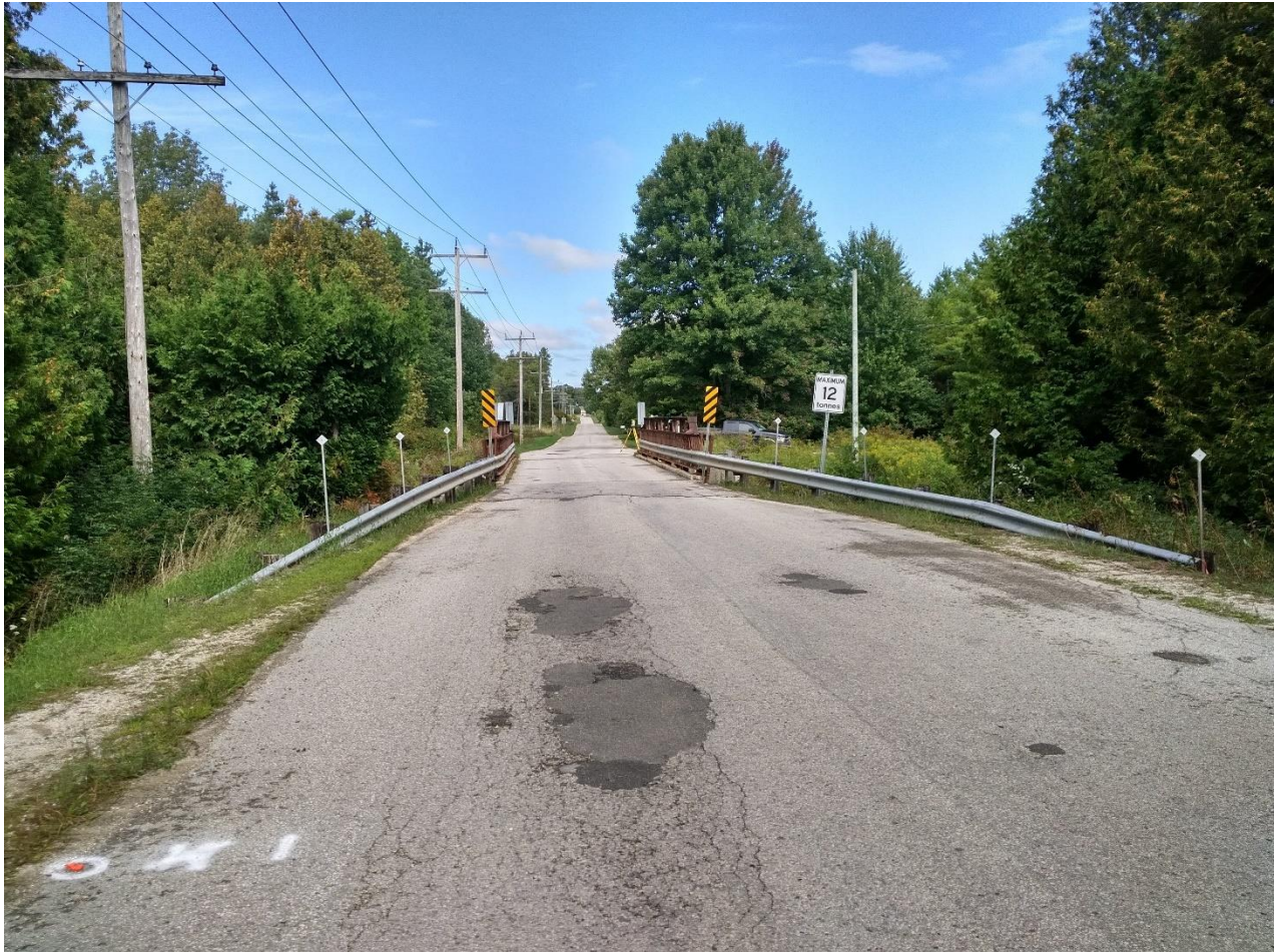
Figure 2.10 Misaligned Approach (looking northbound), September 2019
