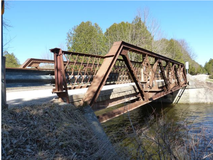
Image 2: Bridge on Normanby-Bentinck Townline over Beatty Saugeen River. Note the similarities in design to those of the Lantz Bridge (HistoricBridges.org)
